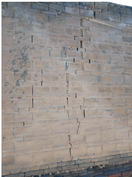
Figure 1. Masonry structure crack 图 1. 砌体结构开裂
