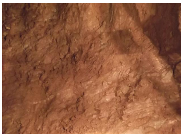
Figure 3. XK28 + 410 rock mass is broken mosaic structure
