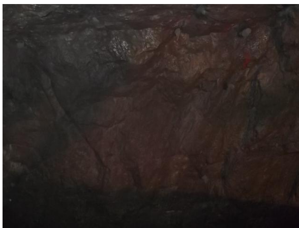
Figure 2. XK28 + 354 rock mass is broken: a complete mosaic structure
