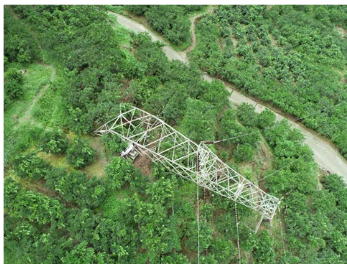
Figure 3. Tower toppling 图 3. 铁塔倾倒
