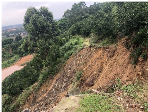
Figure 10. The landslide cut off paths and ditches 图 10. 滑坡切断小道和沟渠
