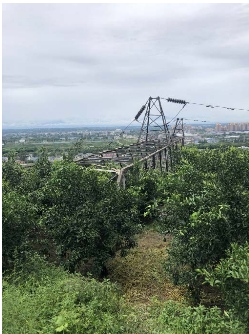
Figure 2. Tower fell down the slope 图 2. 铁塔倒向坡下
