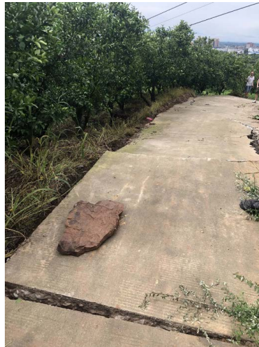
Figure 9. Longitudinal crack 图 9. 纵向裂缝
