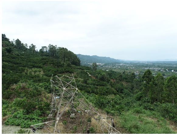
Figure 4. Broken tower at the waist 图 4. 铁塔拦腰折断
