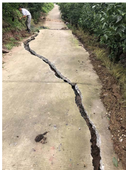
Figure 6. S-shaped crack 图 6. “S”型裂缝
