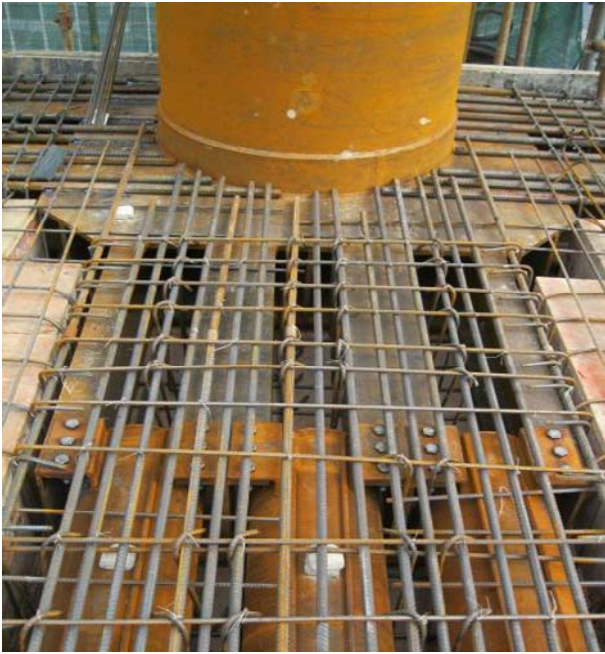
Figure 5. The connection diagram of hollow steel tube and steel column bracket 图 5. 空心钢管与钢柱牛腿连接图
