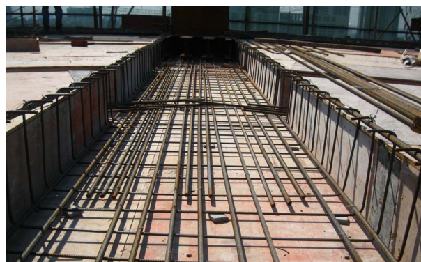
Figure 13. Laid wide flat beam bottom U band and beam bottom bar 图 13. 铺设宽扁梁下部 U 型箍及梁底筋
