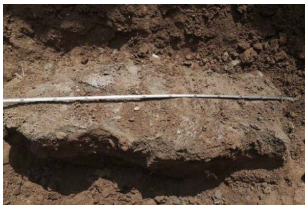
Figure 5. The condition after the excavation of the test section of the Taian Luo Dam reinforcement project
