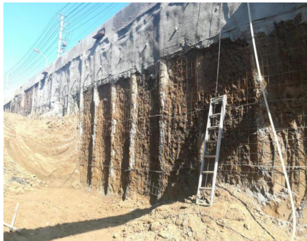
Figure 4. The condition after the excavation of the test section of the comprehensive pipe corridor of Jining station west road
