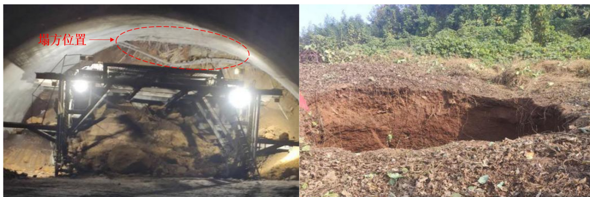
Figure 1. Tunnel face collapse (left) and surface collapse (right) 图 1. 隧道掌子面塌方(左)及地表塌陷(右)
