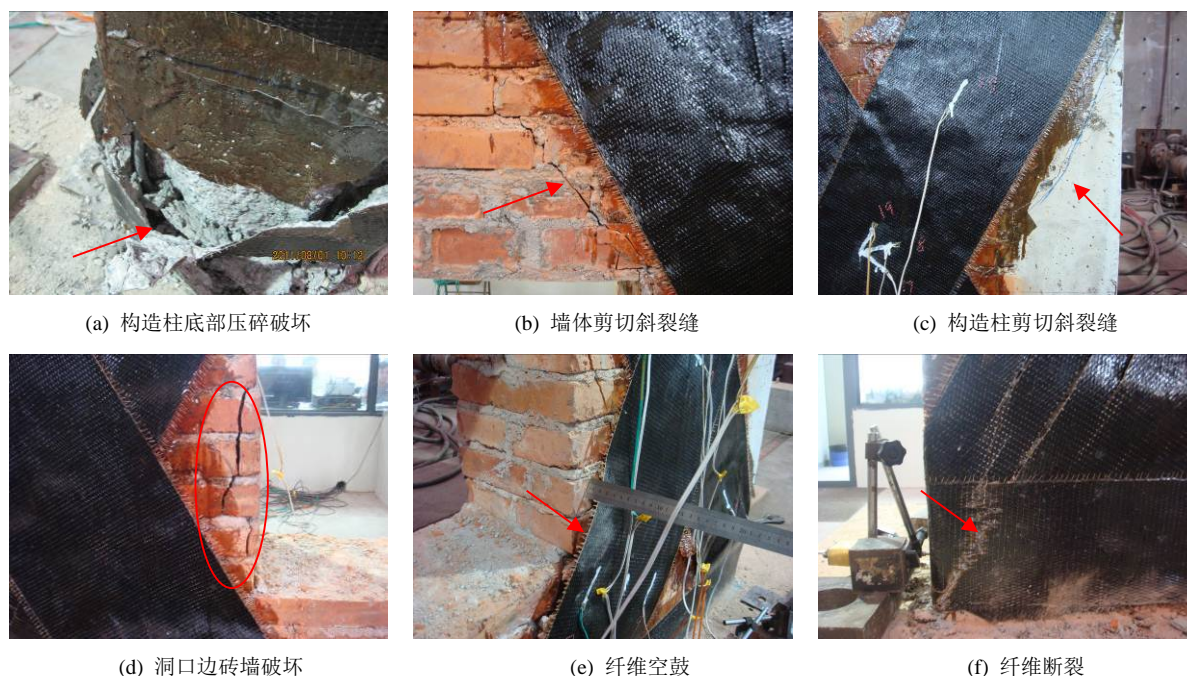
Figure 5. Failure mode of FRP-reinforced masonry wall 图 5. 加固砌体砖墙破坏形态
