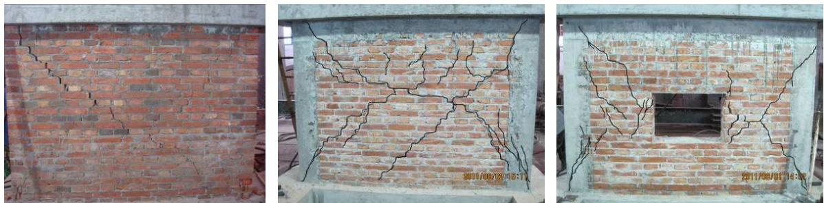
Figure 4. Failure mode of unreinforced masonry wall 图 4. 未加固砌体砖墙破坏形态
