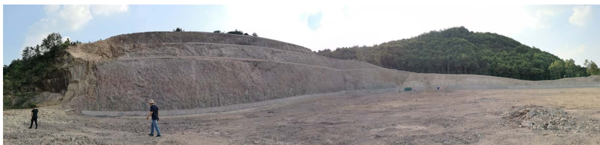
Figure 5. After treatment of Luofangqiao landslide in Yafan Town 图 5. 雅砻镇罗芳桥滑坡治理后现状图
