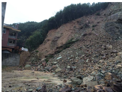
Figure 3. Before treatment of Luofangqiao landslide in Yafan Town 图 3. 雅畈镇罗芳桥滑坡治理前现状图
