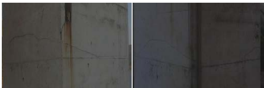
Figure 5. Transverse surface penetrating crack 图 5. 横向贯穿裂缝
