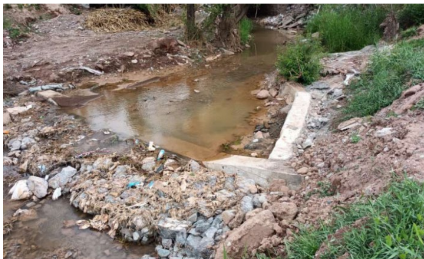
Figure 1. The destroyed retaining wall and the anti-scour wall at small river broke through 图 1. 小型河流穿越挡墙及防冲墙被冲毁
