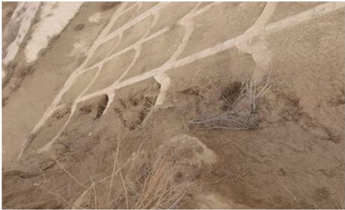
Figure 3. Fracture occurred in the arch lattice and precast concrete block revetment in the collapsible loess section 图 3. 湿陷黄土地区拱形格构与混凝土预制块护岸发生断裂
