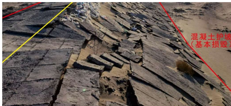
Figure 4. The destroyed concrete windproof and sand-fixing project 图 4. 混凝土防风固沙工程损毁
