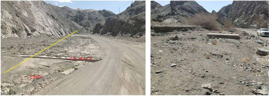
Figure 2. Local slight scouring occurred in the gabion at the section laid along the valley gully 图 2. 山谷河沟敷设段石笼局部发生轻微掏蚀
