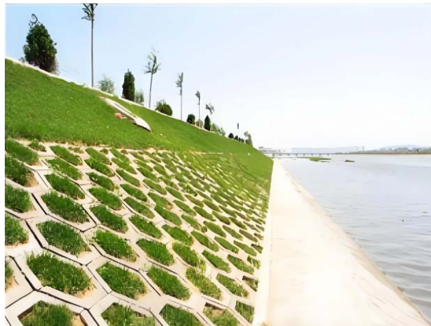
Figure 8. Assembled precast concrete special-shaped blocks + grass planting measures 图 8. 混凝土预制异形块拼装 + 植草措施
