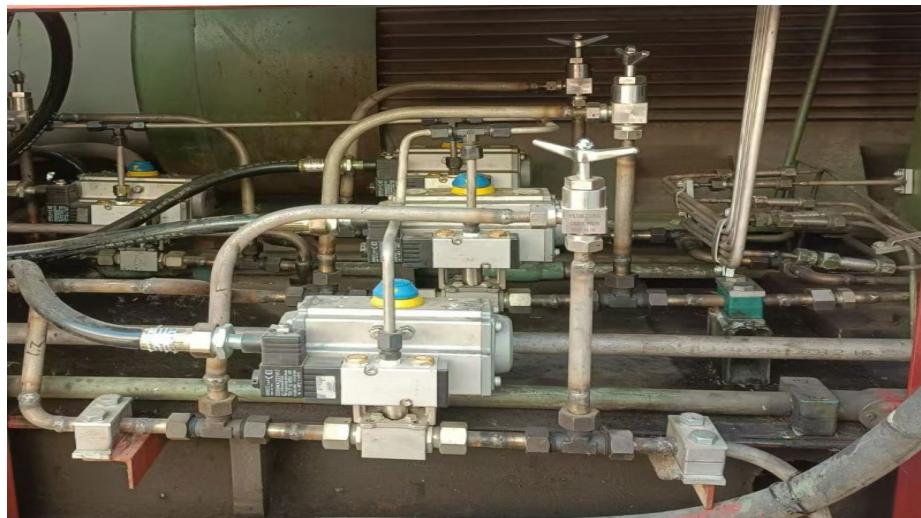
Figure 6. Application of the automatic sewage supply and discharge device 图 6. 自动给排污装置应用
