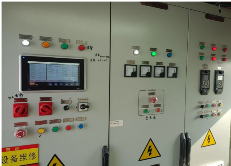
Figure 8. Application of variable-frequency system 图 8. 变频系统应用
