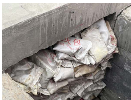
Figure 4. Non-standardized sealing of fireproofing packages 图 4. 防火包封堵不规范
