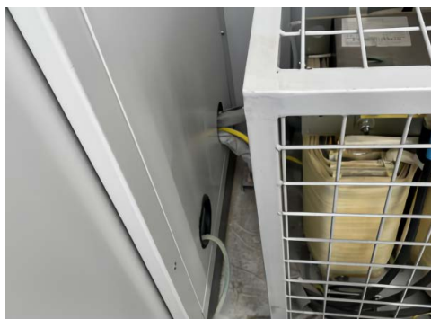
Figure 5. Box change holes without fire blocking 图 5. 箱变孔洞未进行防火封堵
