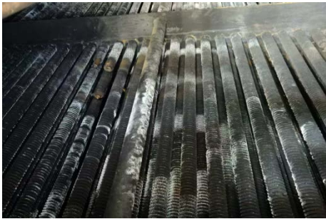
Figure 1. Corrosion and leakage of flue gas heat exchanger 图 1. 换热器腐蚀及泄漏情况
