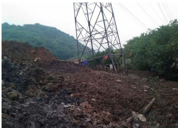
Figure 1. Subsidence caused the tower to tilt 图 1. 沉降引起的铁塔倾斜
