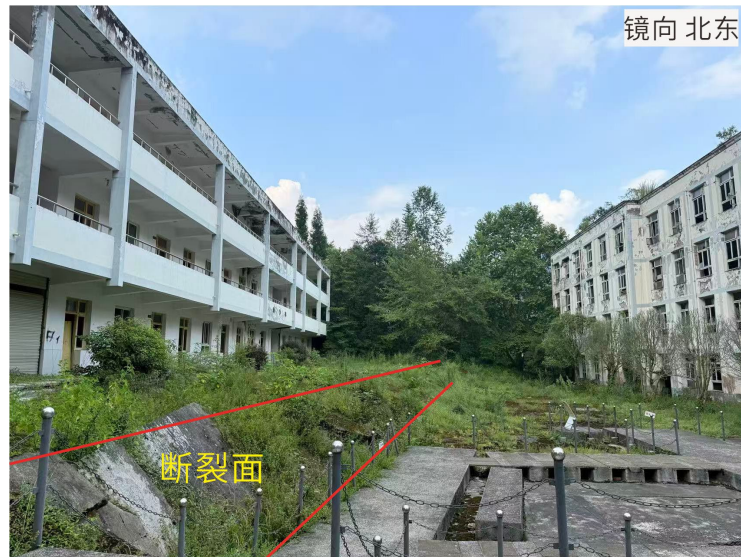
Figure 6. Bailu middle school across the Longmenshan fault 图 6. 龙门山断裂经过白鹿中学
