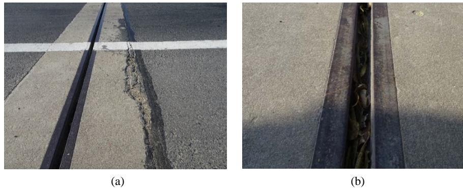
Figure 2. Typical parameters of expansion joint. (a) Local unevenness of anchorage area of expansion joint; (b) Height difference between beams at both sides of expansion joint
