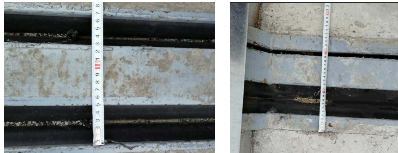
Figure 8. Diseases of expansion joint 图 8. 伸缩缝病害
