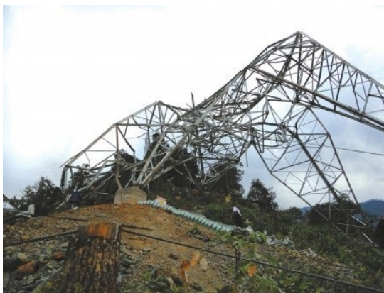
Figure 1. Real scene of damaged transmission towers after the earthquake
