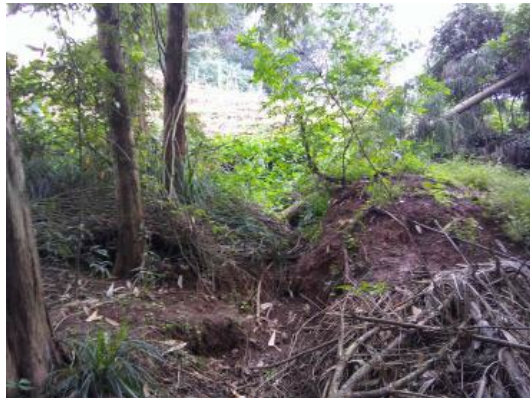
Figure 5. Left boundary (shear crack) 图 5. 左侧边界(剪切裂缝)
