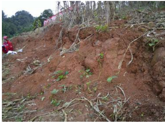
Figure 4. Trailing edge boundary (tension crack) 图 4. 后缘边界(拉张裂缝)
