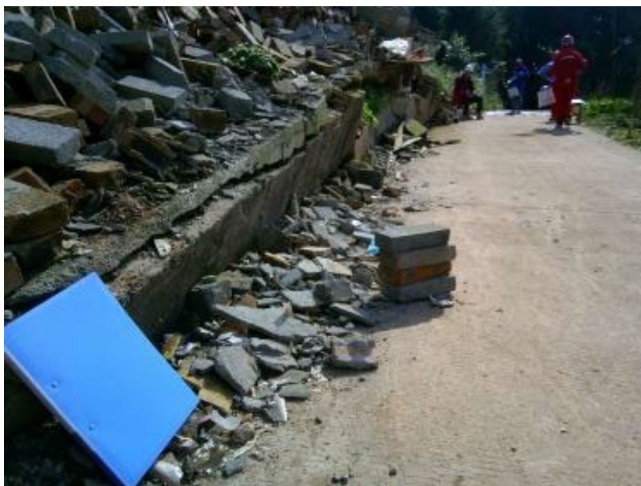
Figure 7. Leading edge boundary (bulge crack) 图 7. 前缘边界(鼓胀裂缝)
