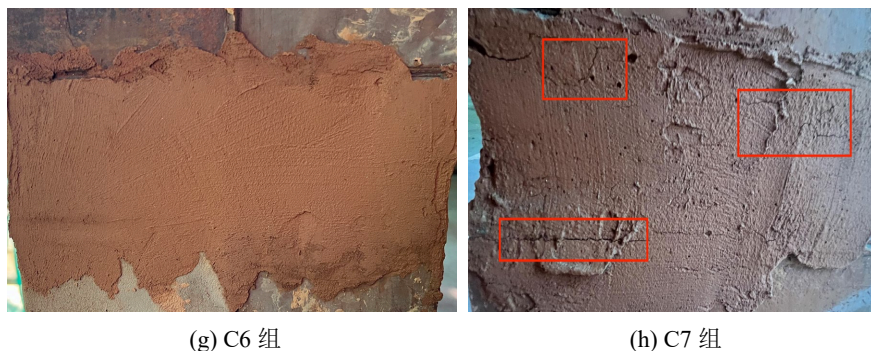
Figure 5. Mortar cracking (construction site) 图 5. 砂浆开裂情况(施工现场)
