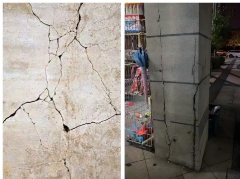
Figure 1. Cracks in the wall and columns
