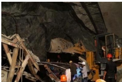
Figure 1. Collapse of the arch crown at the tunnel
