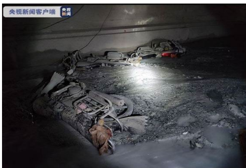
Figure 2. Water and mud inflow at the tunnel
