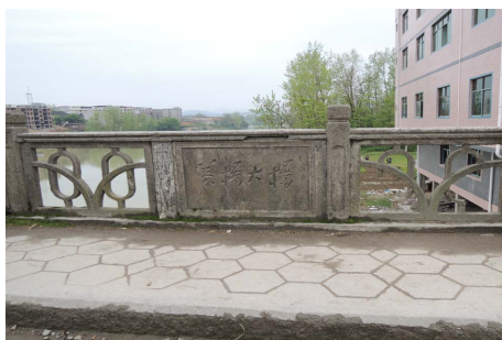
Figure 11. Severe damage to the guardrail and corrosion of the reinforcement
