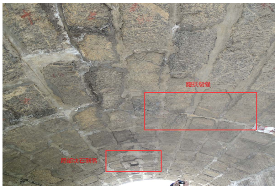
Figure 8. Abdominal arch cracking, with some boulders falling off locally 图 8. 腹拱开裂、局部块石脱落
