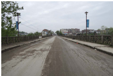
Figure 10. Damaged bridge deck pavement and water accumulation
