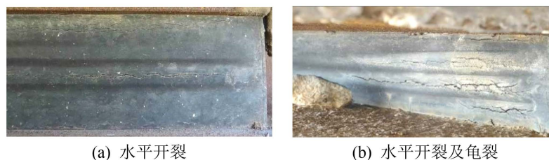
Figure 2. Cracking of plate rubber bearing
