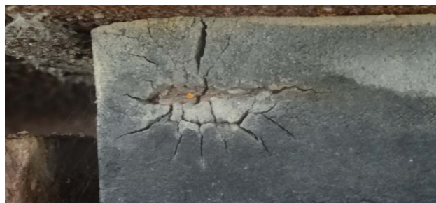
Figure 3. Exposure of steel sheet inside the plate rubber bearing
