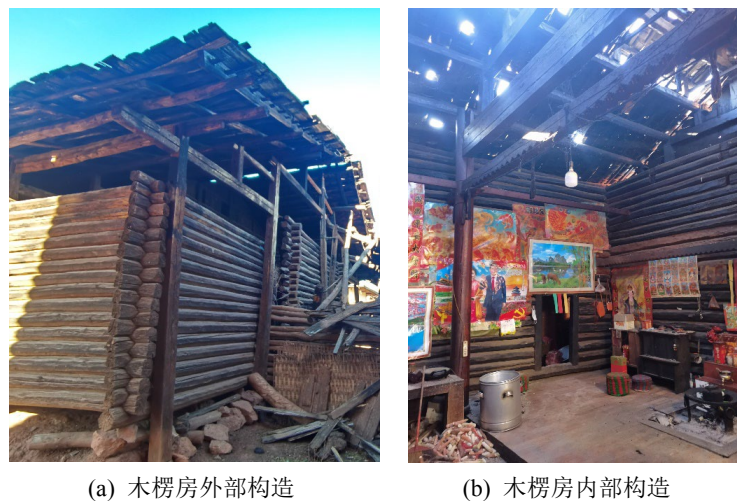
Figure 2. Structural diagrams of single-story Mosuo wooden log houses 图 2. 单层摩梭木楞房构造图
