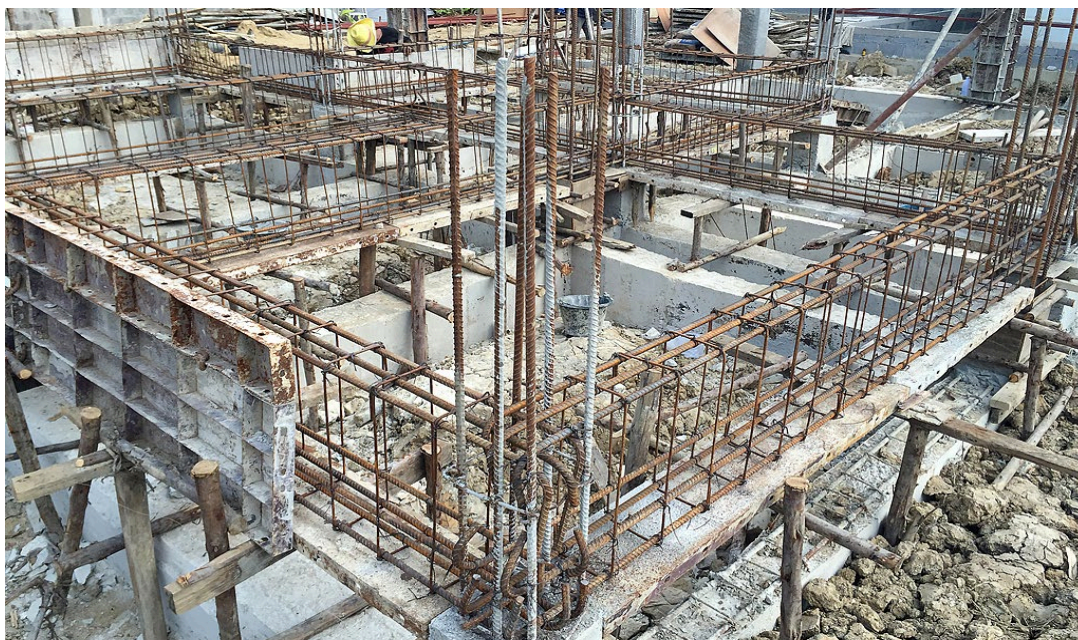
Figure 5. Reinforcement binding construction for steel-concrete frame beam-column joints 图 5. 钢筋混凝土框架梁柱节点钢筋绑扎施工
