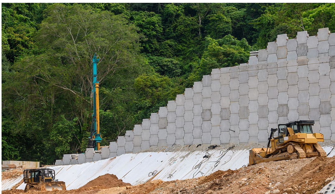
Figure 6. Example of a reinforced retaining wall project 图 6. 加筋挡土墙工程示例
