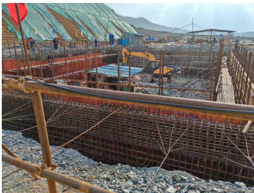
Figure 1. Construction site drawing on the start of excavation 图 1. 开挖初期施工现场图
