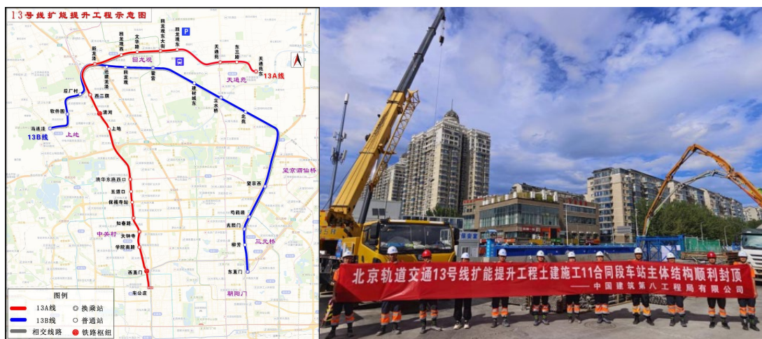
Figure 4. The route and construction site of the Beijing Metro Line 13 renovation project 图4. 北京13号线改造工程线路及工地现场
