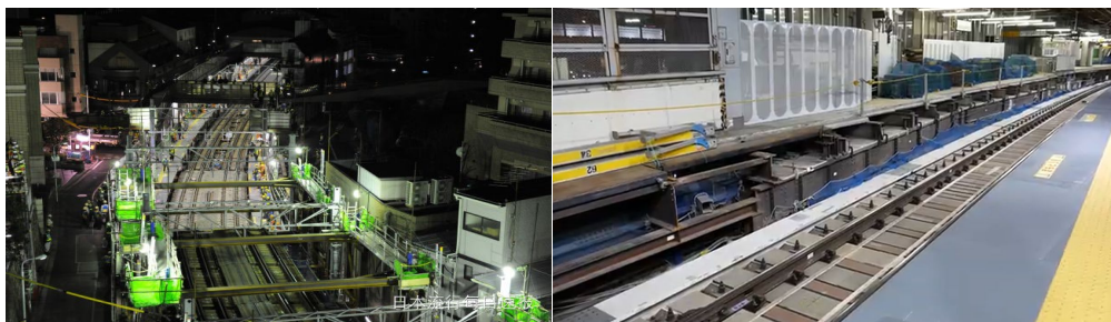
Figure 3. Photos before and after the construction of the Shibuya Station Project in Tokyo 图 3. 东京涩谷站再开发项目施工前后相片
