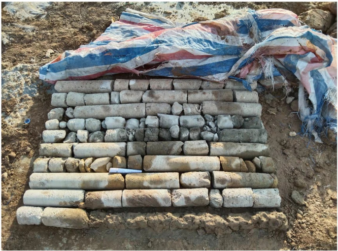
Figure 2. Unqualified strength and integrity of pile-body 图 2. 桩身强度、完整性不合格
