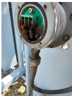
Figure 1. Shows the rusting condition of the main transformer body pressure surge relay 图1. 主变本体压力突发继电器锈蚀情况
