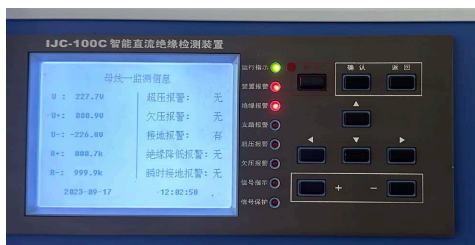
Figure 2. DC insulation detection monitoring information 图2. 直流绝缘检测监测信息
