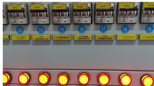
Figure 4. The 17th branch circuit breaker 图 4. 第 17 支路空开
