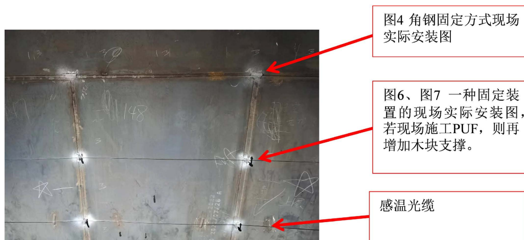
Figure 8. The actual installation diagram of the temperature-sensing optical cable on the inner wall of the outer tank 图 8. 外罐内壁感温光缆实际安装图
