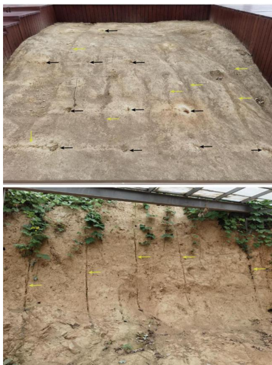
Figure 3. Erosion by splash detachment of raindrops and surface runoff at Laohuling Site. (a) The effects of the temporary rainshed. Black and yellow arrows indicate puddles caused by splash detachment of raindrops and shallow ridges caused by surface runoff, respectively. (b) Shallow ridges of Laohuling Site, showed by yellow arrows
