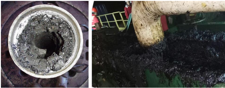
Figure 3. Pipeline events caused by asphalt (Right picture is M-B-41 precipitated asphalt) 图 3. 沥青造成的管线事件(右图是 M-B-41 析出沥青)
