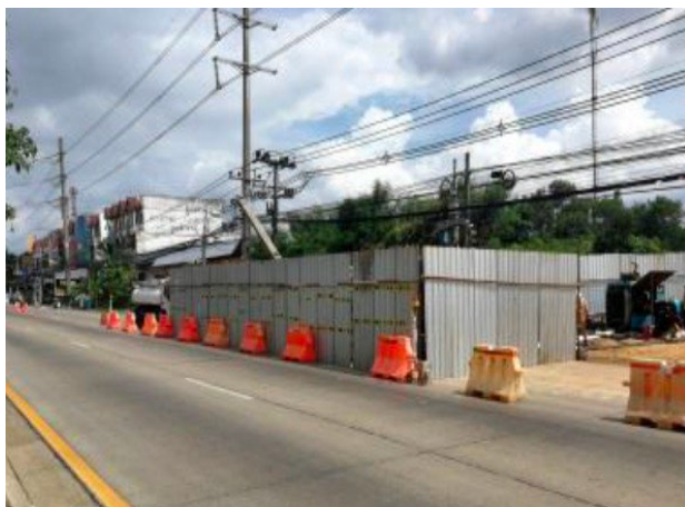
Figure 4. Sound insulation barrier 图 4. 隔音屏障
