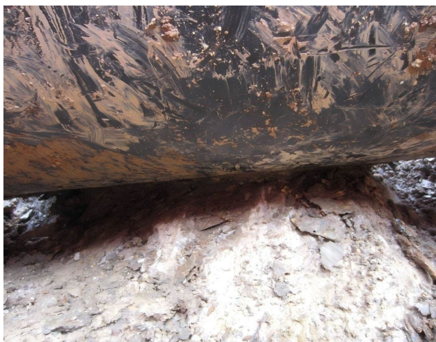
Figure 3. Boulder at the 6 o'clock position under pipeline 图 3. 管底 6 点位置孤石
