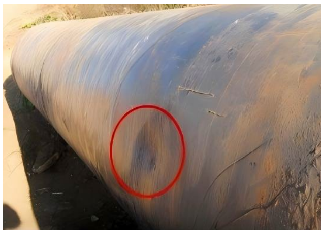
Figure 5. Dent on pipeline outer surface 图 5. 管道外表凹陷
