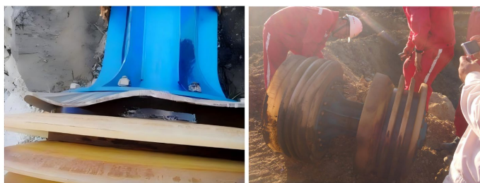
Figure 1. Picture of the serious deformation of gauging disc
