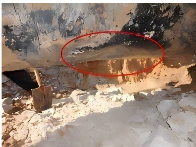
Figure 4. Serious deformation at 6 o'clock of pipeline bottom 图 4. 管道 6 点位置严重变形
