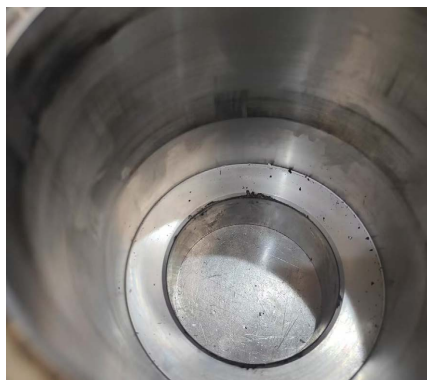
Figure 11. Photograph of cavitation on the valve seat 图 11. 阀座气蚀图
