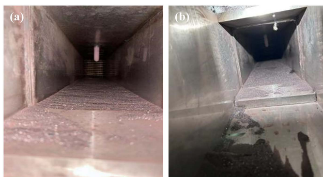
Figure 9. Ash distribution in the duct at front of the heat exchanger specimen (a) and ash distribution at the position of the heat exchanger specimen placed (b)
