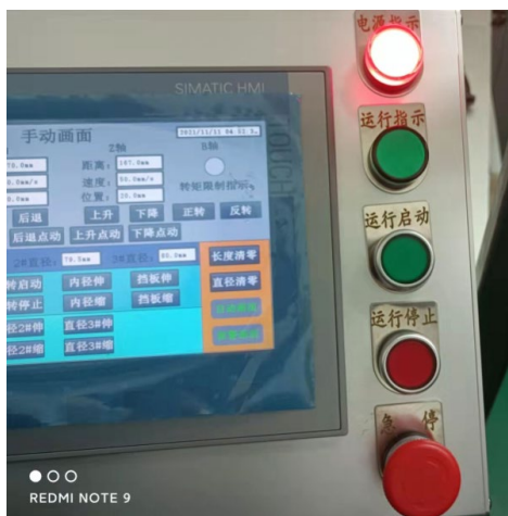
Figure 19. Emergency stop button on the device operation panel 图 19. 设备操作面板急停按钮
