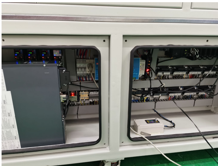
Figure 18. Equipment electrical cabinet 图 18. 设备电气柜
