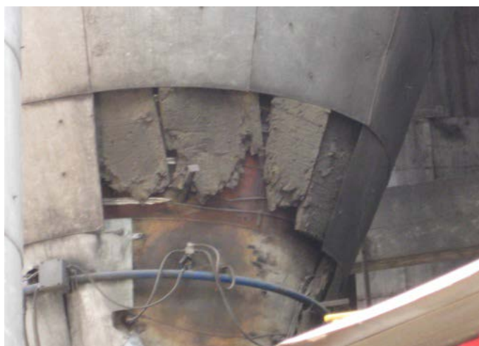
Figure 3. The phenomenon of rock wool falling off in the preheating furnace
