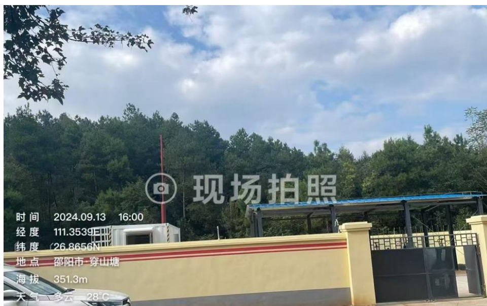
Figure 3. Valve chamber C on a Shaoyang natural gas pipeline segment 图 3. 邵阳某天然气管段阀室(阀室 C)
