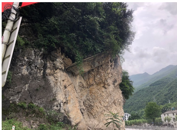
Figure 1. Dangerous rock mass W1, photo
