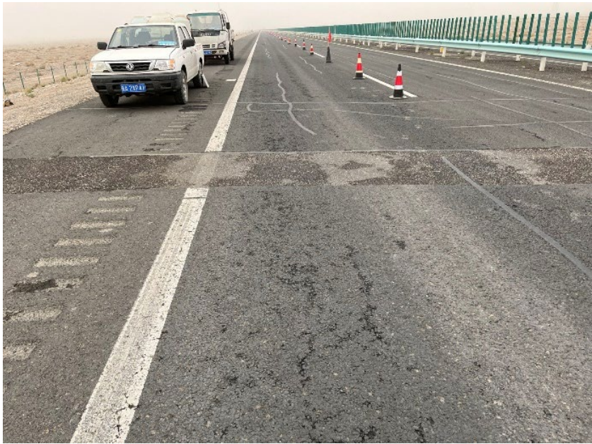
Figure 2. Upheaving distress along the Aksu-Kashi section of the G30 12 Expressway 图 2. G30 12 阿克苏至喀什高速公路拱胀病害
