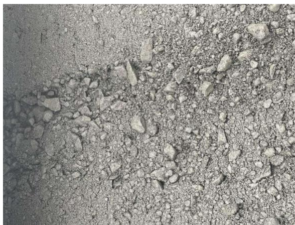
Figure 8. Coarse aggregate segregation 图 8. 粗集料离析
