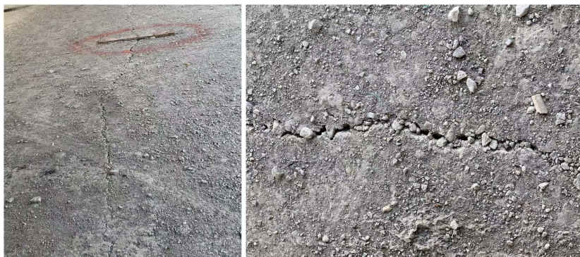
Figure 4. Cracks on the surface of the cement-stabilized base layer
