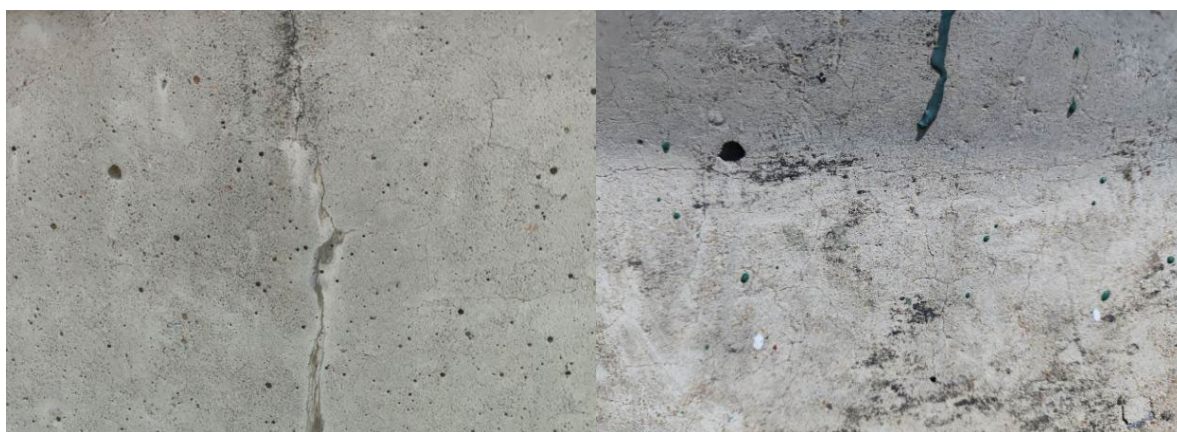
Figure 2. Cracks and reticular cracks
