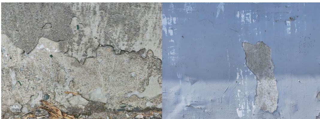
Figure 9. Coating spalling 图 9. 涂层剥落
