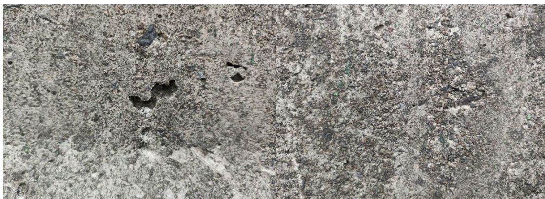
Figure 4. Dissolution pits and surface sanding
