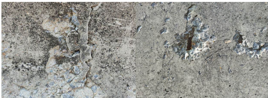
Figure 3. Surface spalling and exposed reinforcement
