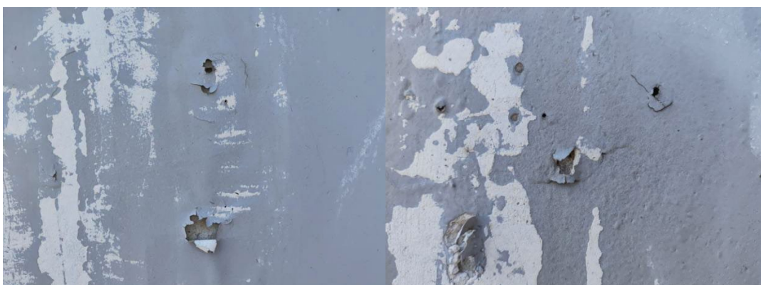
Figure 10. Coating blistering 图 10. 涂层鼓包、起泡
