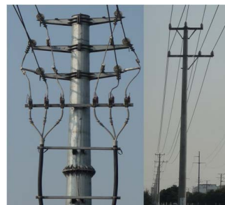
Figure 3. The arrangement of the lines (As shown in the left graph line 124 is arranged in the left and line 123 is arranged in the right of the No.1 tower. The phase-sequence is arranged up and down like BAC; As shown in the right graph line 124 is arranged in the bottom and line 123 is arranged in the top of the No.2 tower. The phase-sequence is arranged left and right like CBA)
