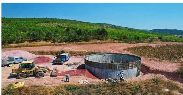
Figure 1. Construction site of circular reservoir in mountainous area 图 1. 山区圆形蓄水池施工现场
